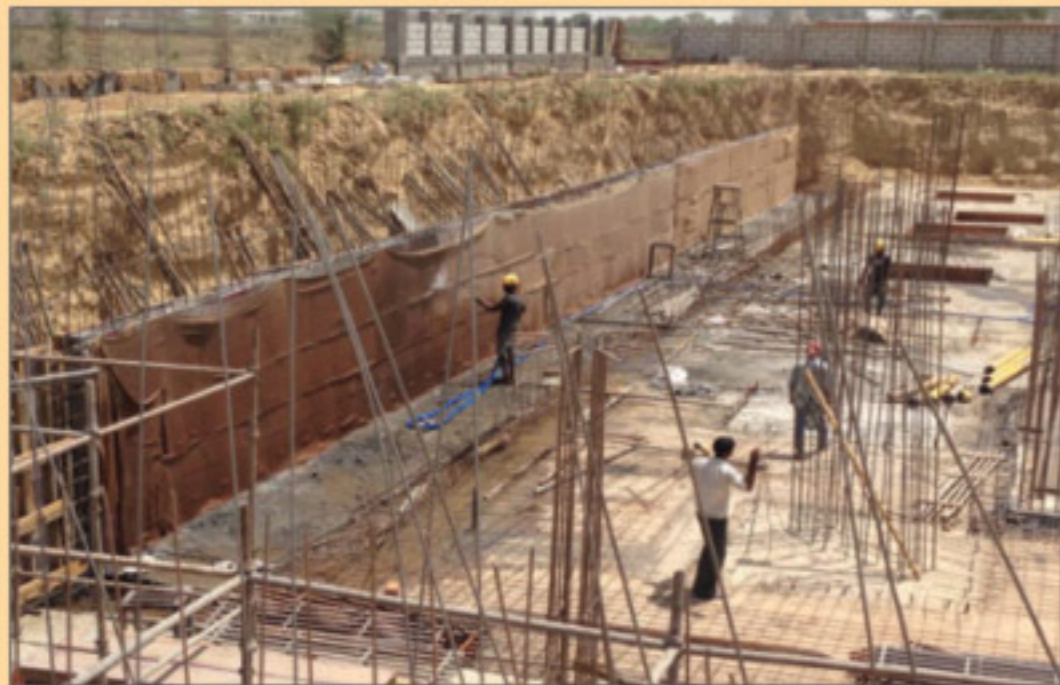
Basement retaining wall RCC 1st lift (2400 mm height) towards north east side
